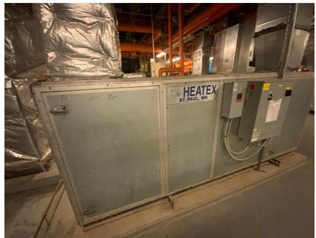
24 - ENERGY RECOVERY UNIT
