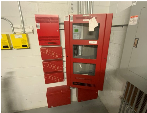
29 - FIRE ALARM PANEL
